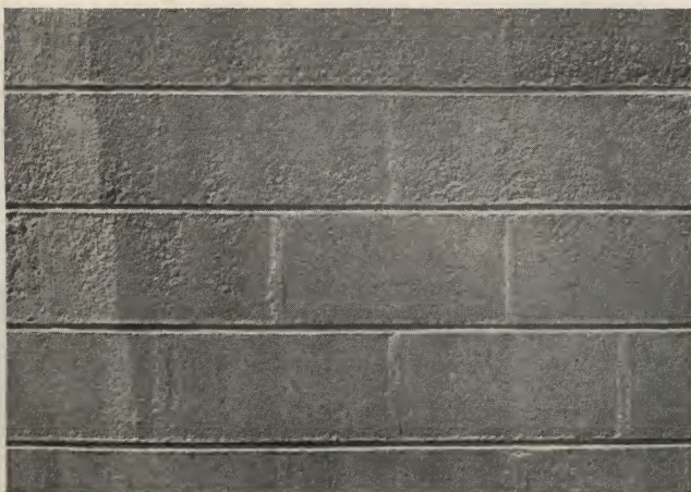
3—Close-up of wall section shows how vertical joints are obscured and horizontal joints brought out. Wall is finished with two coats of portland cement paint.
